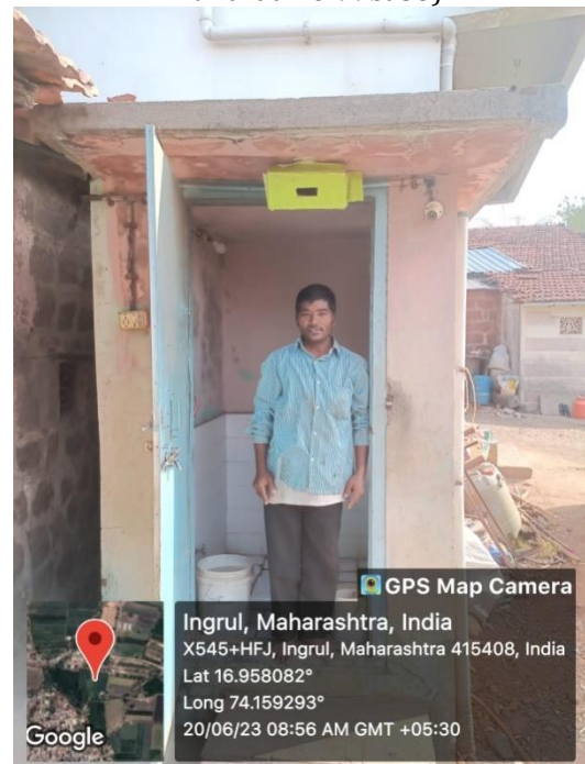
Sensor Attached in the toilet
